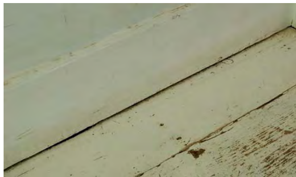
This pic & below: Rattling sash windows and draughty floorboards in the TV room
